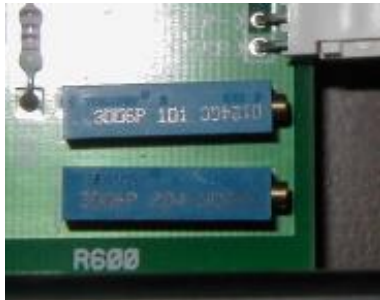
Advanced Controller – the zero potentiometer is the closest to the front
